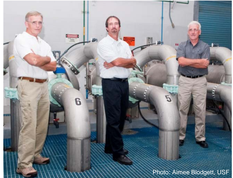
From left to right: Tom Burke - City Engineer, Paul Stanek - Water Division Director, and Ken Stidham - Wastewater Division Director
